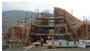
Draft tube forms currently under construction behind the project offices near the Trail Airport
